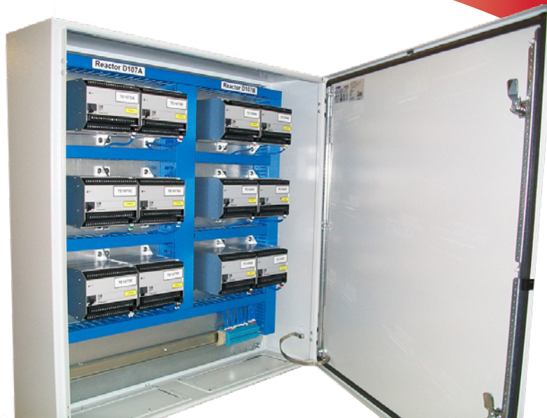
Figure 2. Remote I/O was local I/O reconfigured and housed to be remotely installed from its corresponding controller/CPU.
