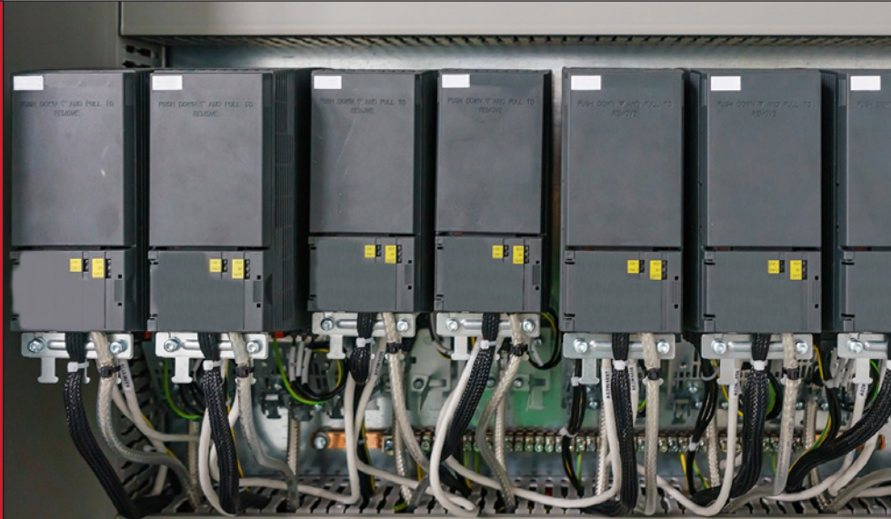
Figure 1. Local I/O is typically collocated within the same cabinet.
