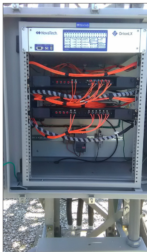
Figure 1. Typical communication and automation processor RTU panel with direct video monitor, input/output (I/O), panel metering, and intelligent electronic devices.
