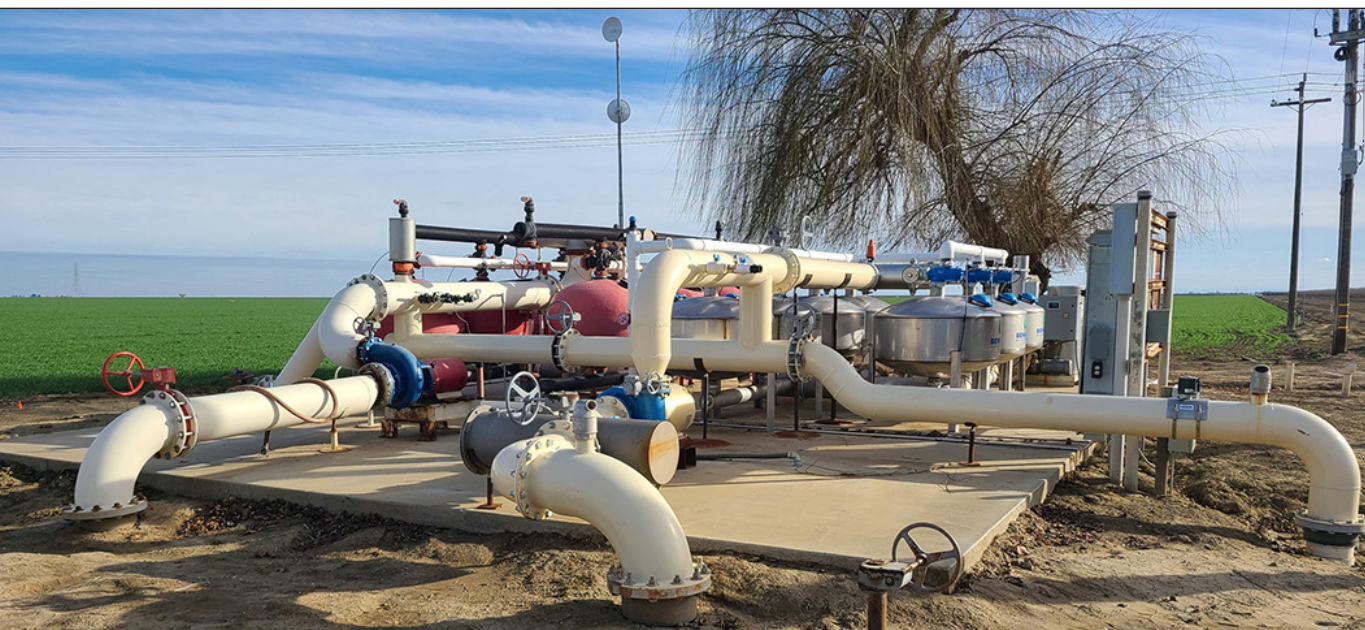
Figure 3. Azcal filter stations typically serve multiple crops in fields of various sizes.
