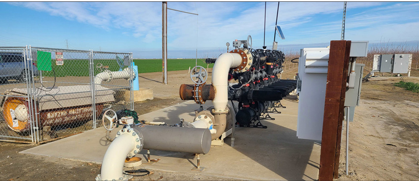
Figure 1. All Azcal wells and irrigation filter stations are equipped with VFDs and flowmeters.
