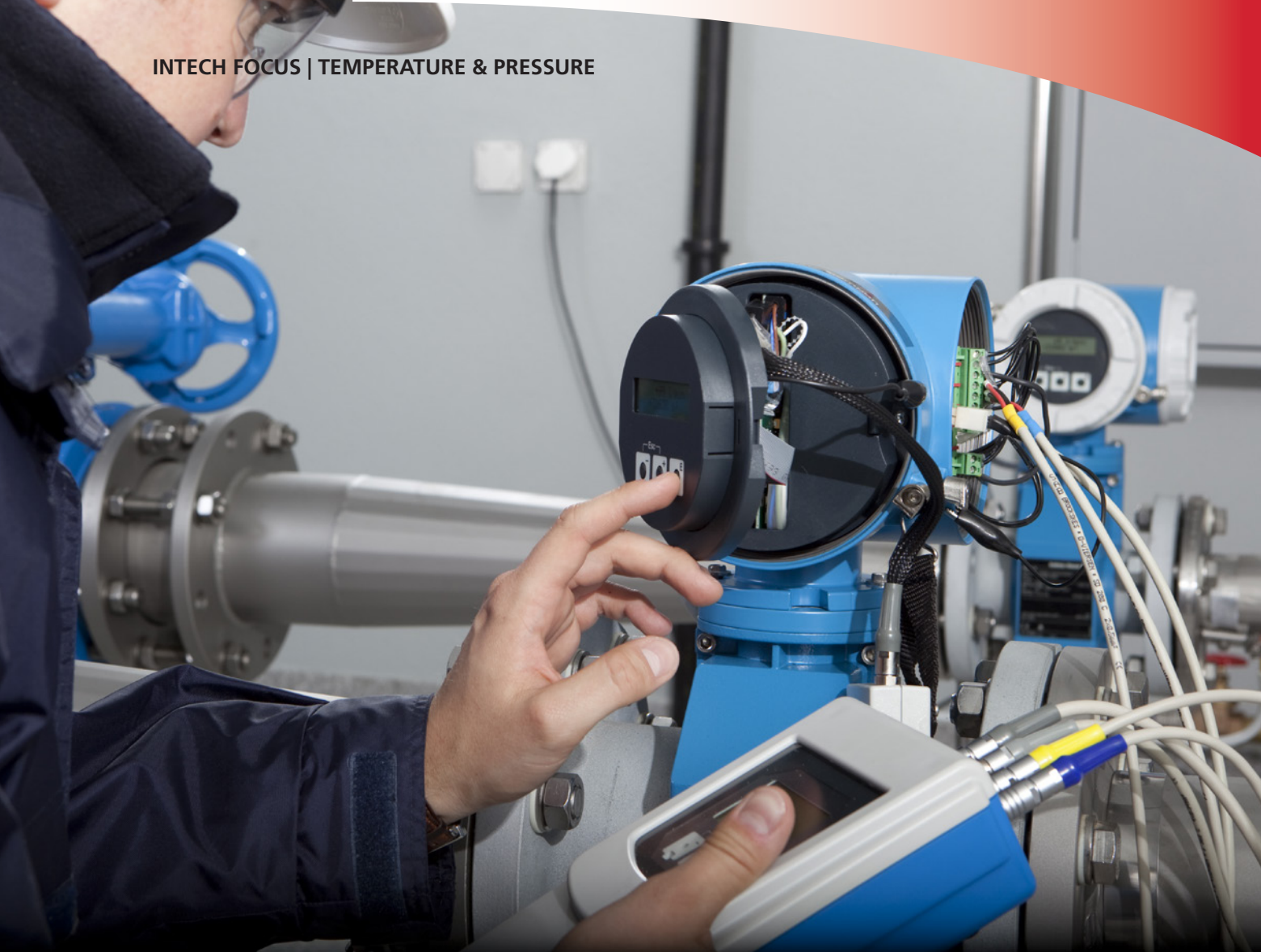
Figure 1. An individual technician can evaluate instruments one by one, but this manual approach cannot keep up with a large population of field devices.
