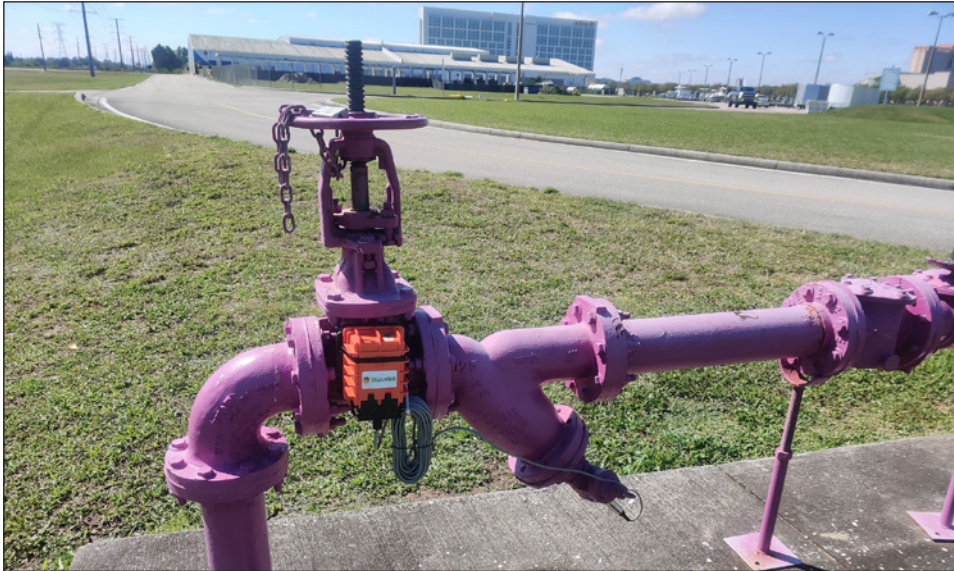
Figure 1. Ayyeka AI-enabled edge devices, such as this unit that tracks reclaimed water use in Orange County, Fla., use ultra-long-life bobbin-type \text{LiSOCl}_2 batteries to monitor hard infrastructure, delivering enhanced data intelligence by recognizing patterns, detecting anomalous events, providing real-time reporting, and enabling predictive modeling.
